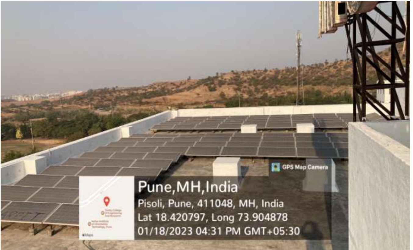
Rooftop solar power generation system
