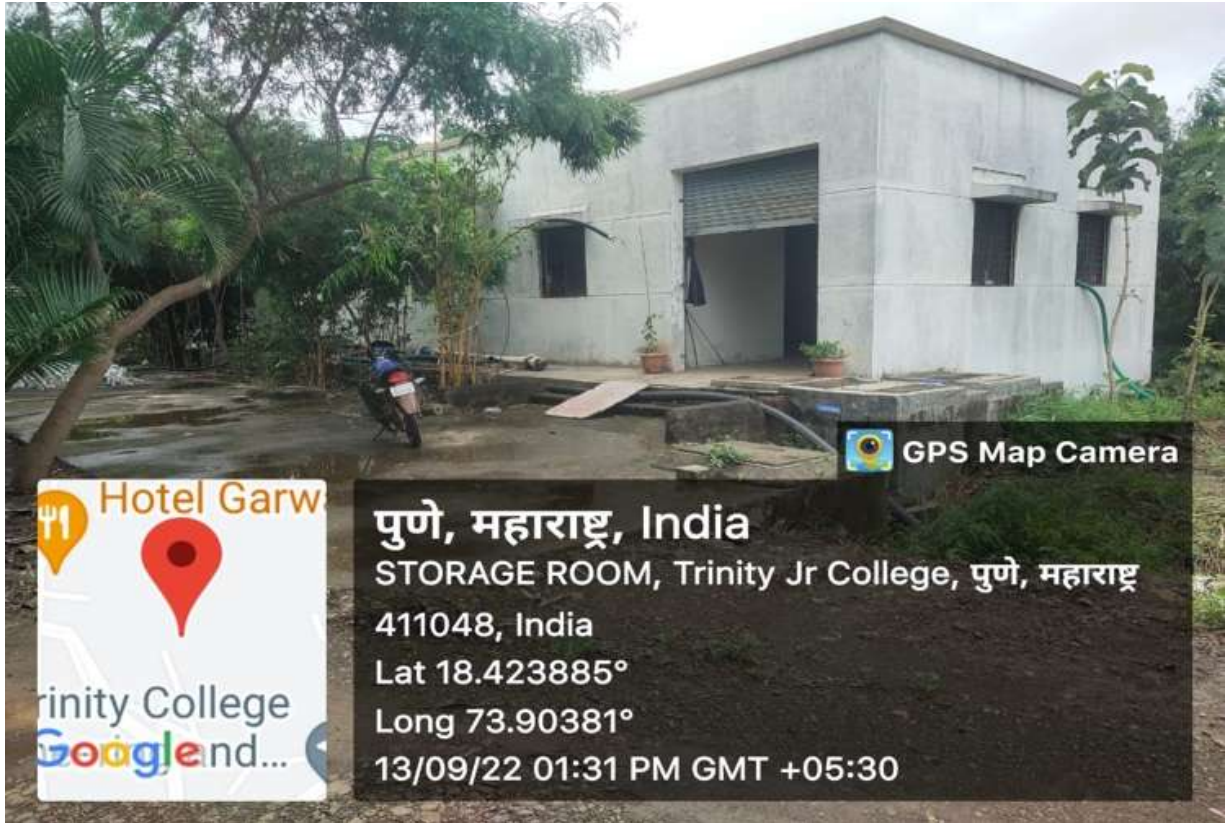
Sewage Treatment Plant (STP)
