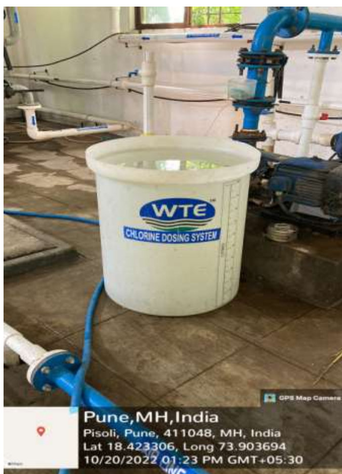
Chlorine dosing system in STP
