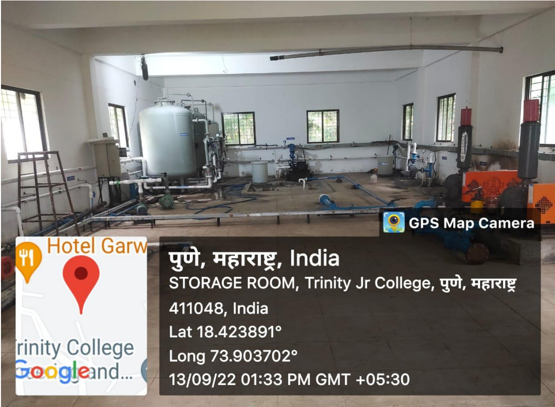
Sewage Treatment Plant (STP)
