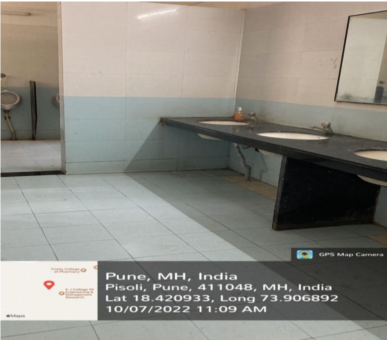
Skid resistant flooring in toilet block
