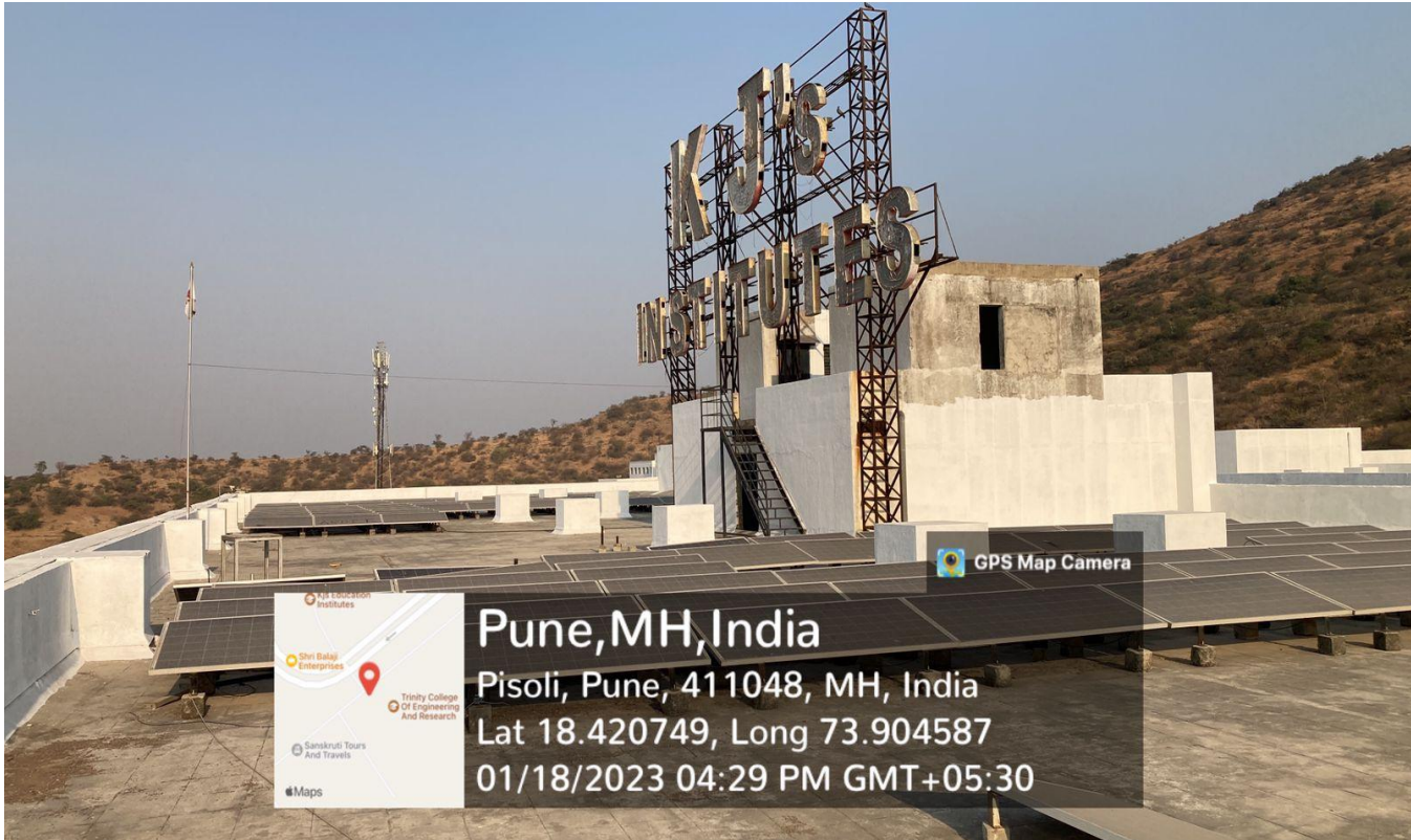
Rooftop solar power generation system
