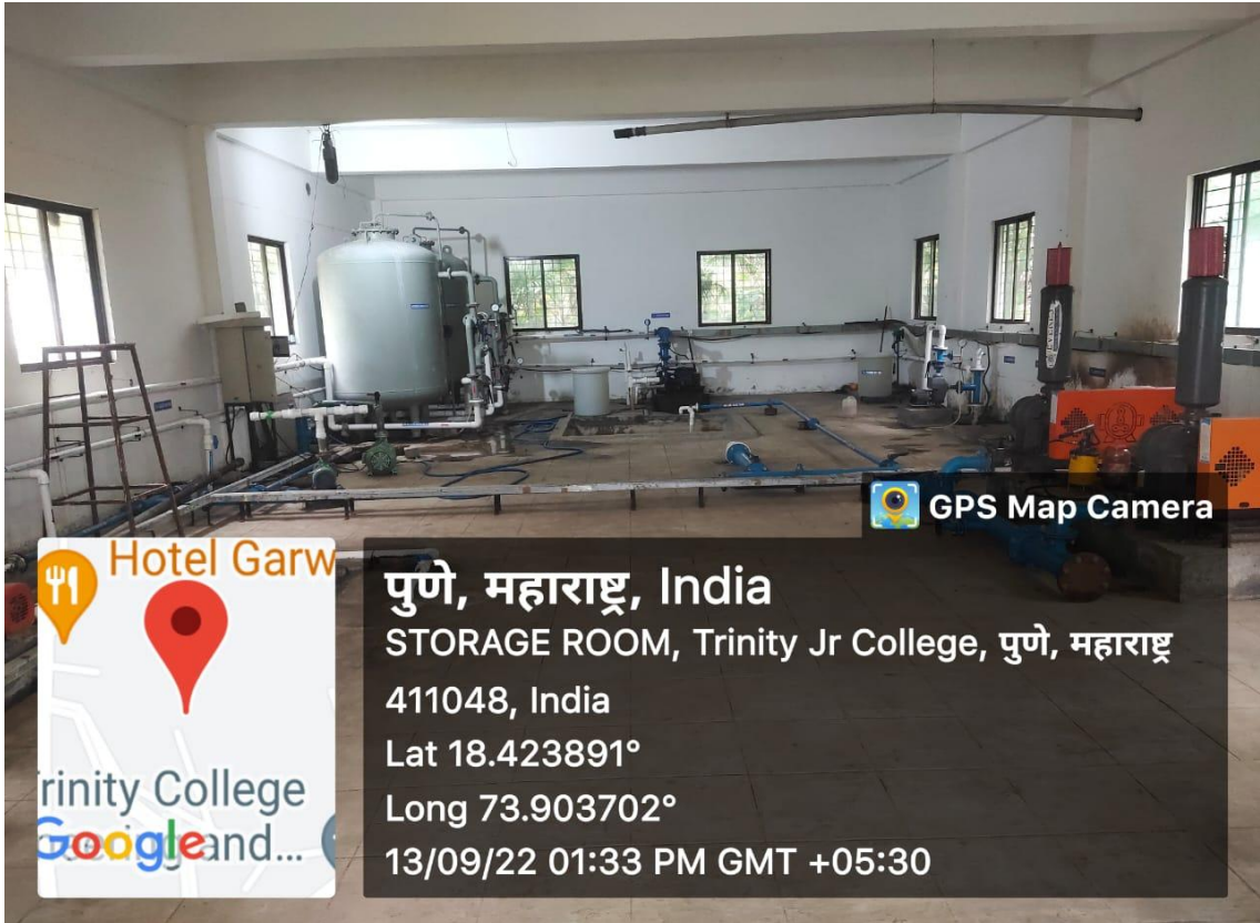
Sewage Treatment Plant (STP)
