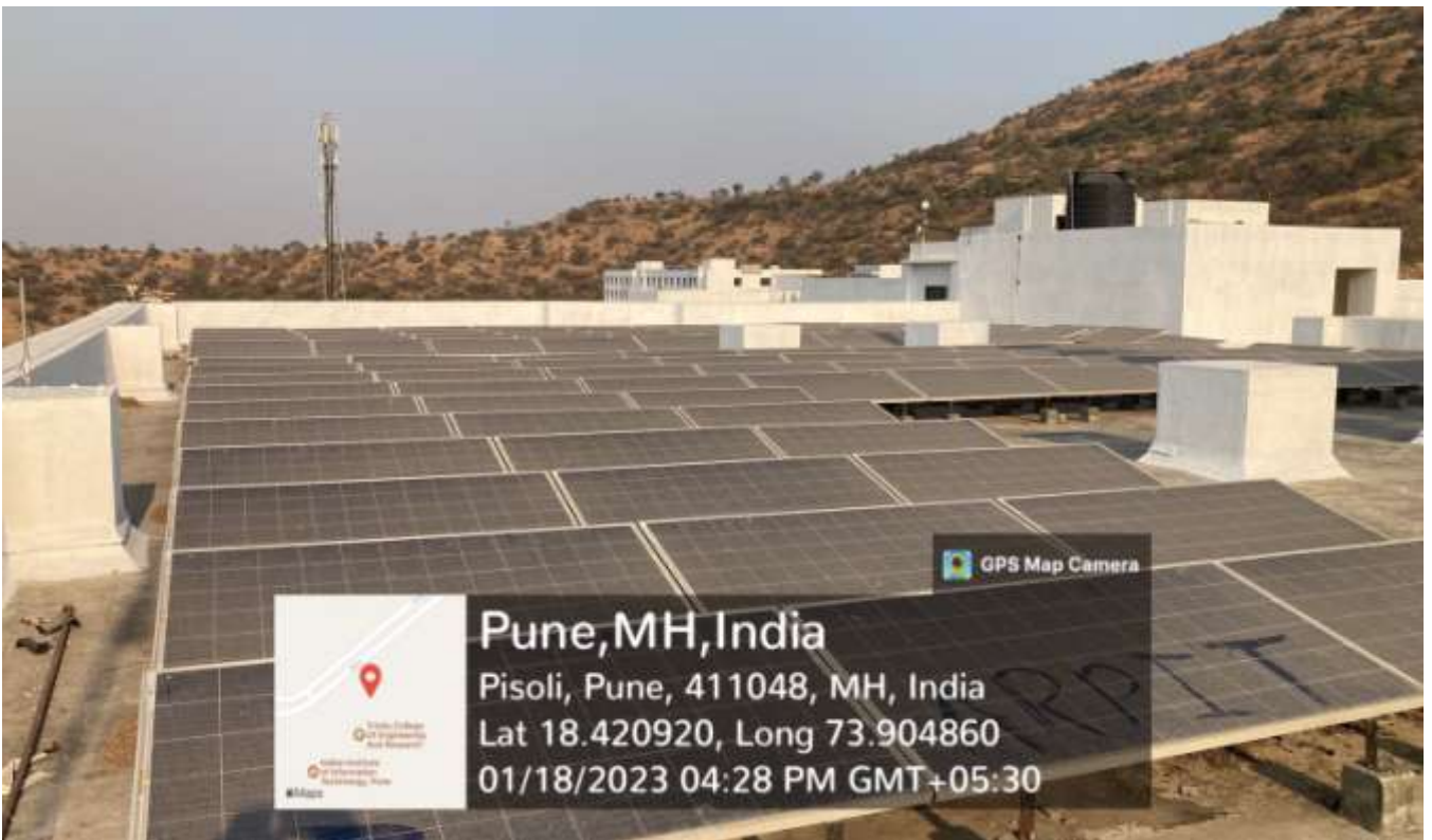
Rooftop solar power generation system
