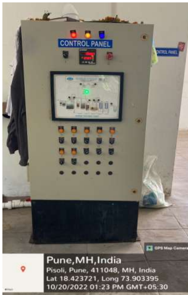
Control Panel of STP
