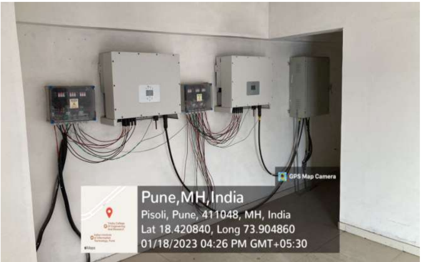
Generated solar energy distribute to main grid
