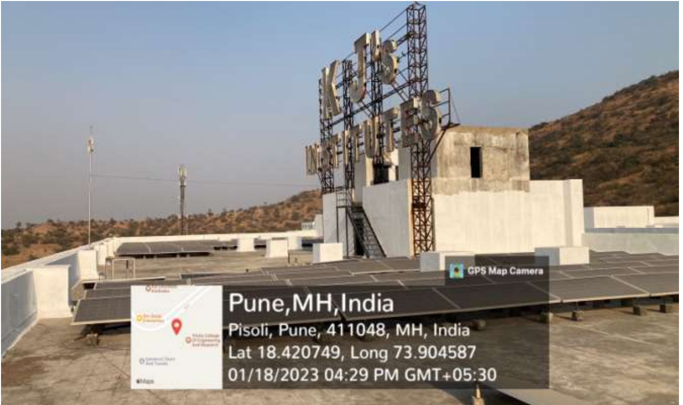
Rooftop solar power generation system
