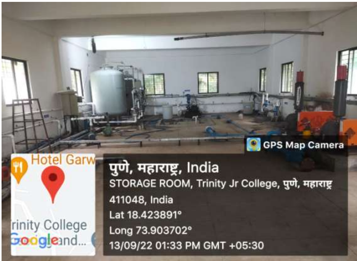
Sewage Treatment Plant (STP)
