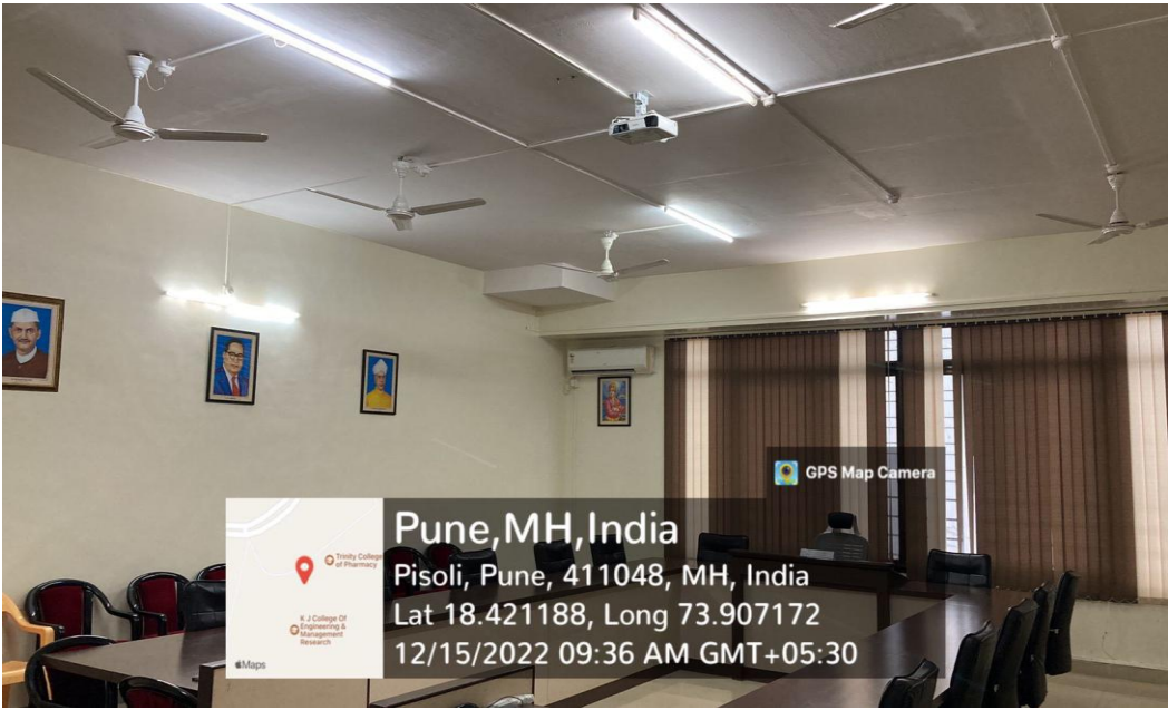
LED lights in board room
